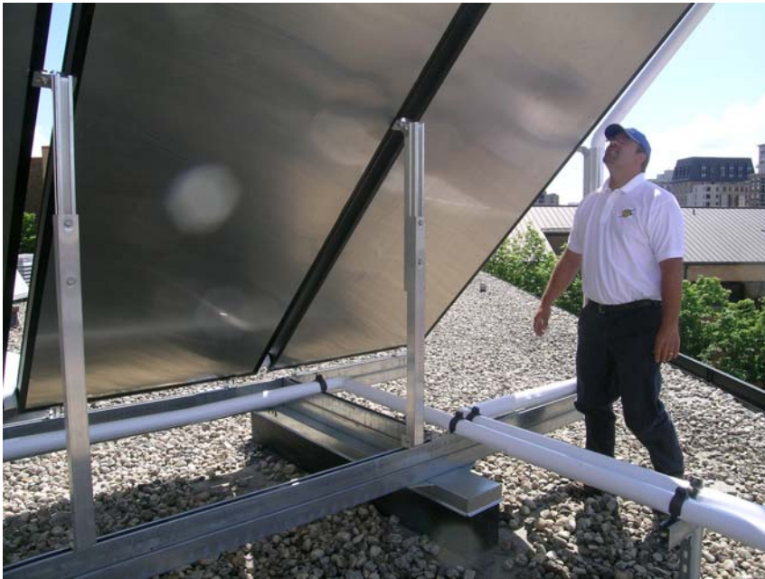
H&H installer Shawn Young on the roof of Fire Station No. 1, Madison
