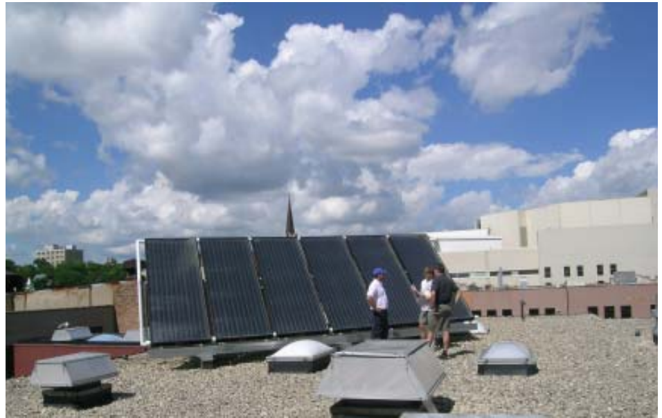
Solar installer Shawn Young (H&H Solar), RENEW's Michael Vickerman, and the City of Madison's Kay Schindel (left to right) inspect the solar hot water system on Station No. 1 with the downtown Madison skyline in the background.
