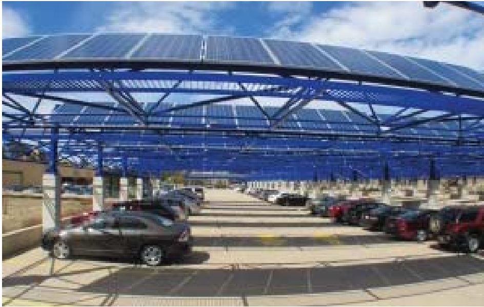
With 1,300 solar panels covering Epic System’s parking lot in Verona, the installation ranks third in the state among similar projects. Photo by Joe Plautz, J.H. Findorff
