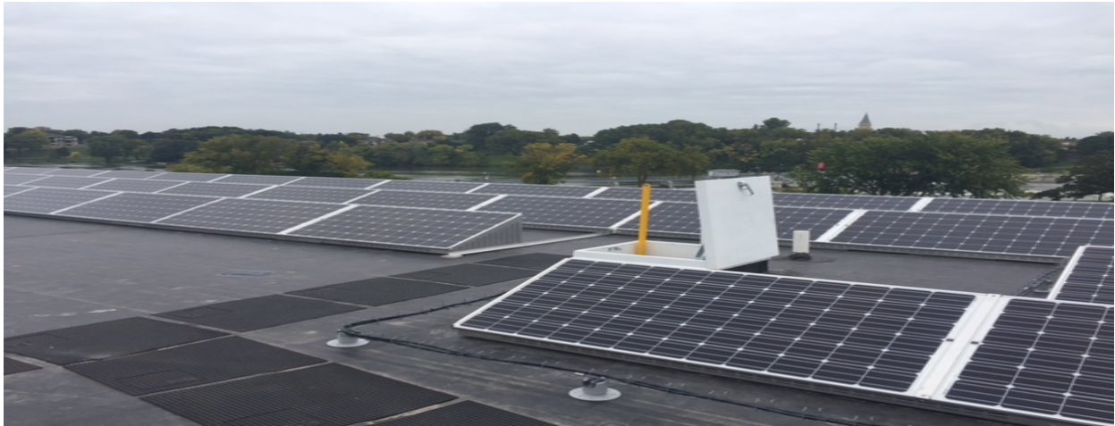
80 kWdc South Wing (looking North)
