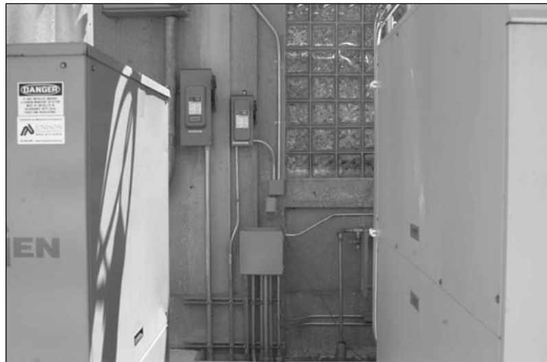
480 v Interconnection point requiring proper clearance
