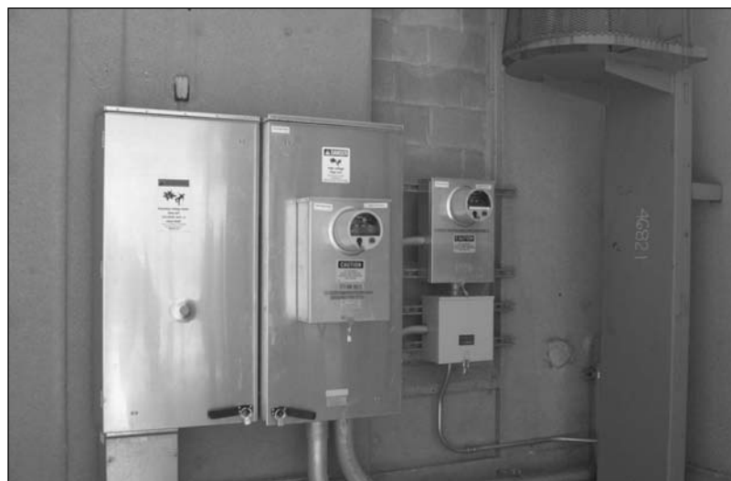
Typical utility metering installation
