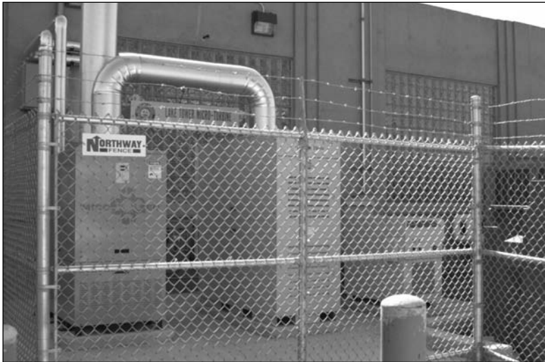
Typical CHP Installation
