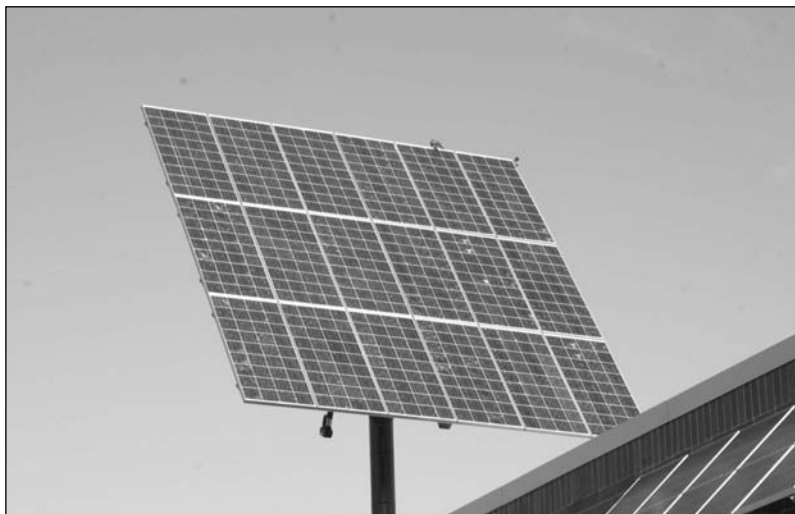
Typical Solar-Photovoltaic Installation
