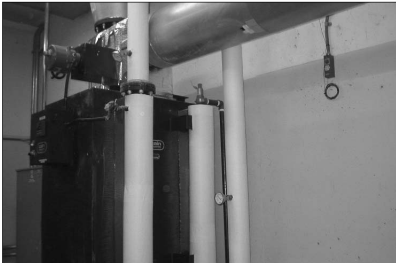
Exhaust heat from MicroTurbines being transferred to hot water in a heat exchanger
