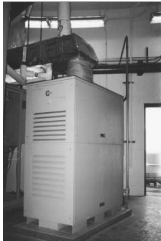
Exhaust heat being recovered from Capstone MicroTurbines
