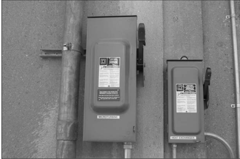
Typical 480 v manual disconnect with a visible open
