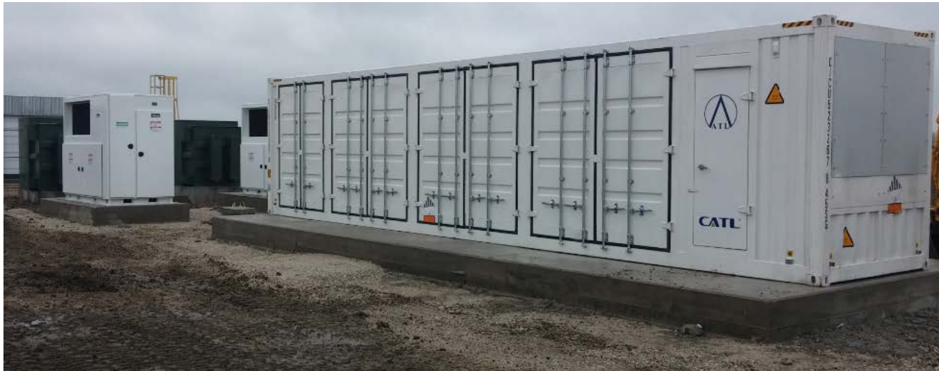
Grand Ridge IV Exp, 3MW, 1.5MWh
