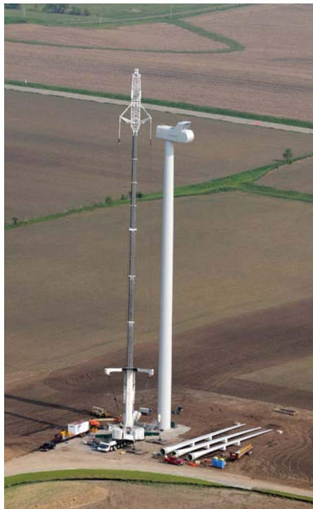
Turbine erection commences on the first of 90 turbines at Glacier Hills Wind Park in Columbia County. (Photo courtesy of We Energies)
